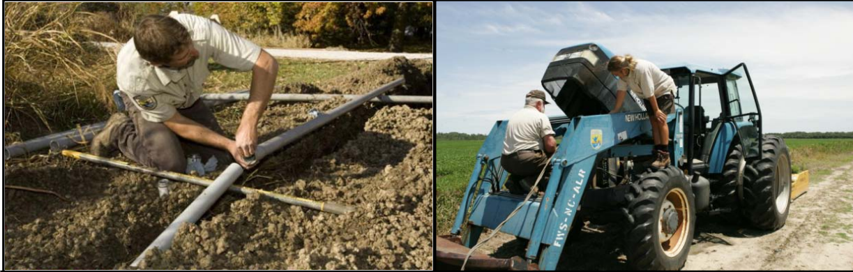
Refuge Maintenance Support and Annual Maintenance include funding for refuge staff to maintain and repair assets and equipment necessary for wildlife habitat management activities.
